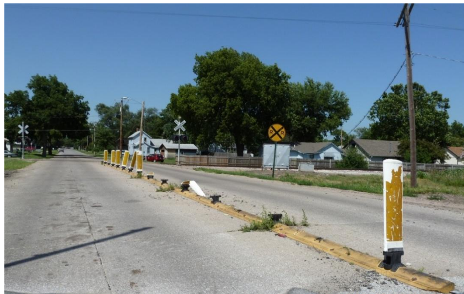
FIGURE 3.2 Condition of the median barriers prior to maintenance
